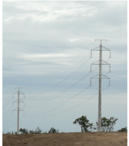
The proposed Yuleba North to Clifford Creek and Dinoun South transmission lines (the subject of this newsletter) is expected to look similar to this existing line located near the Warrego Highway between Condamine Power Station and the Columboola Switching Station (near Miles).
