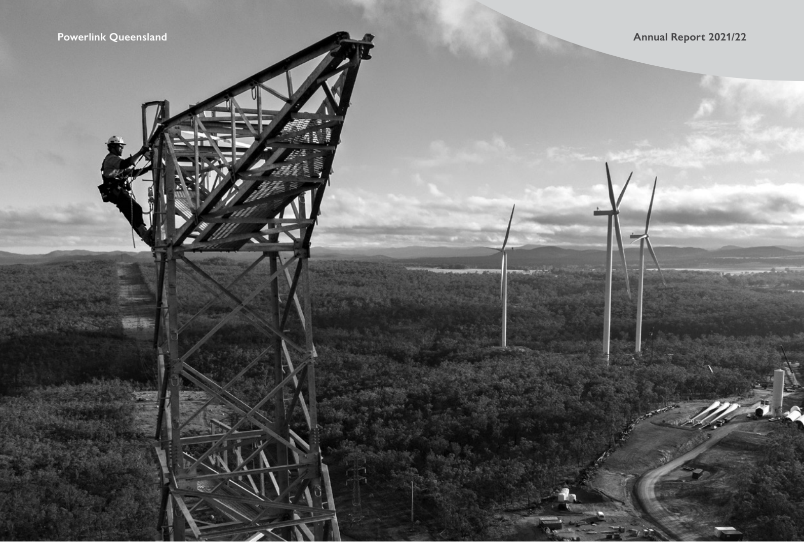
Climbing the tallest transmission towers on our network, built for the Kaban Green Power Hub Connection Project.
