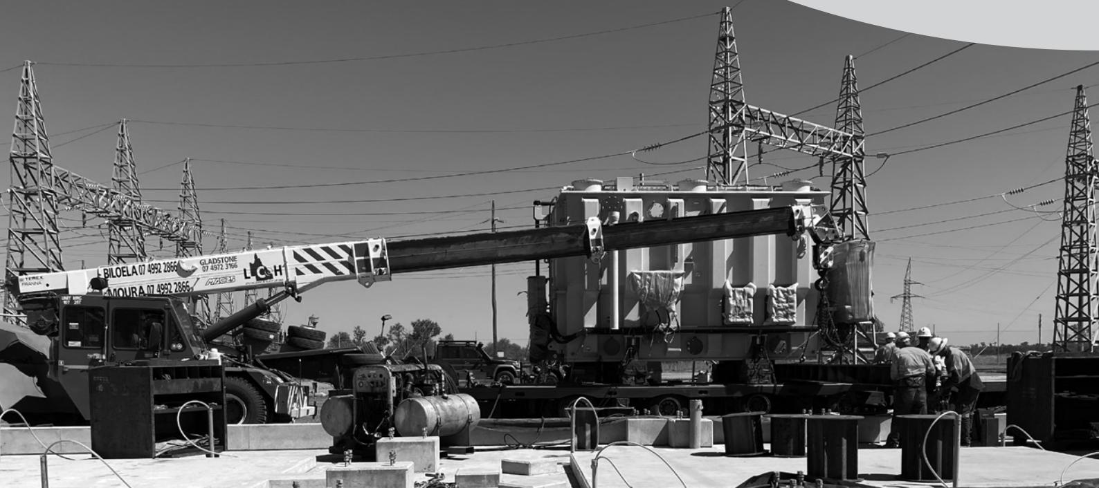
A transformer being installed at Lilyvale Substation to further bolster power supply in Central Queensland.
