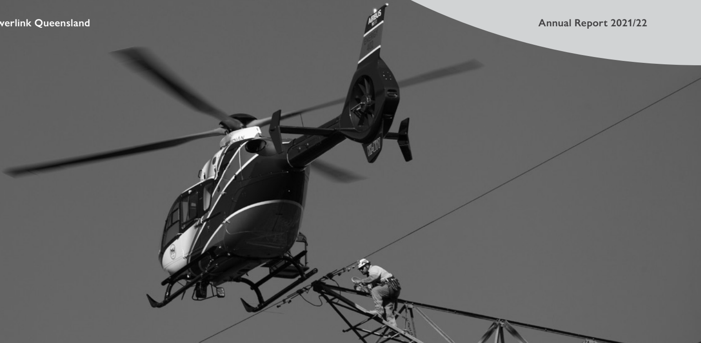
Specialised maintenance work taking place on the Bayview Heights to Davies Creek transmission line.
