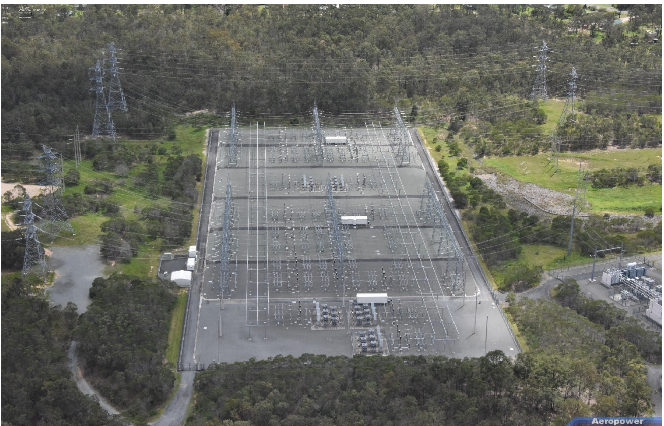
Pictured: Greenbank Substation, south of Brisbane
