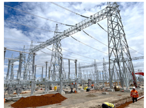
Tummalville Switching Station site.
