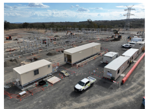
MacIntyre Switching Station site.
