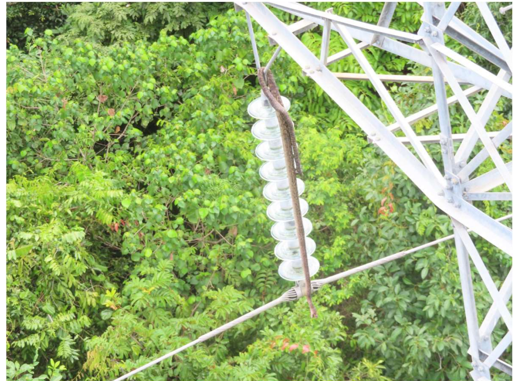
Photos of 132kV tower with Snake who caused fault, and loss of supply to Edmonton and Innisfail substations
