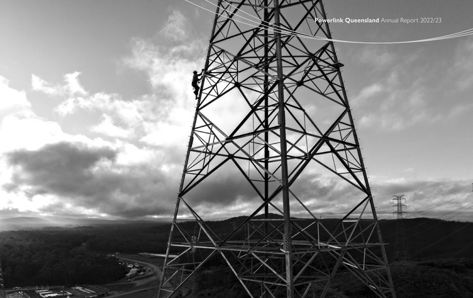
Undertaking final tower assembly work as part of delivering on the Queensland Energy and Jobs Plan.
