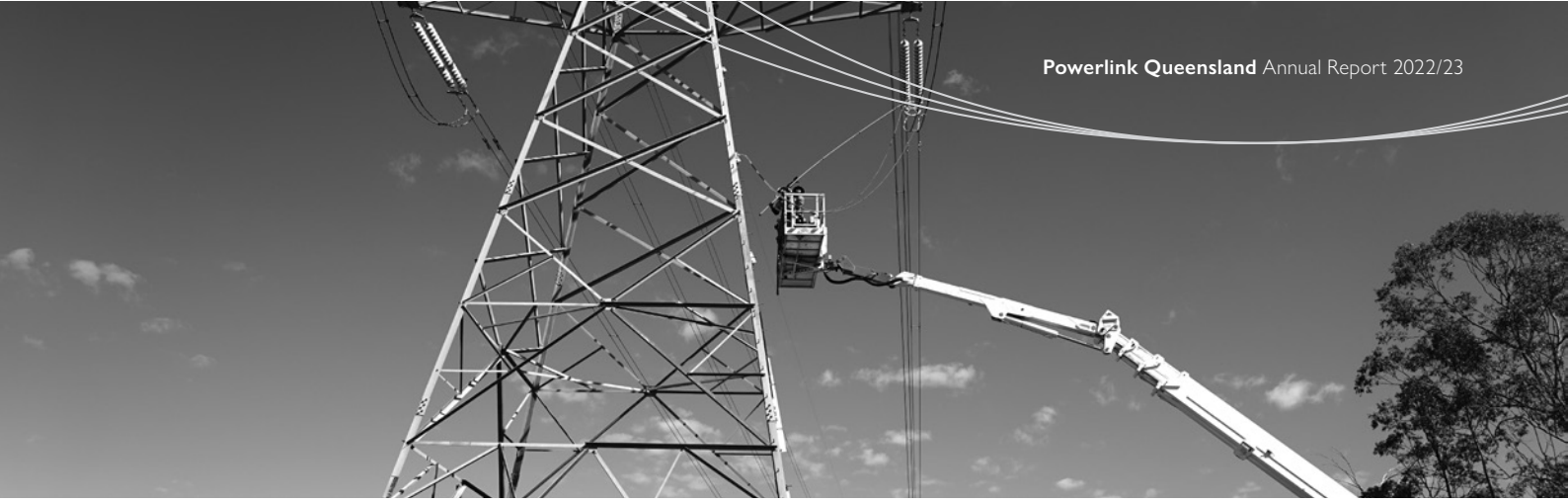
Undertaking insulator replacement work as part of our maintenance program on the Belmont to Bundamba transmission line.
