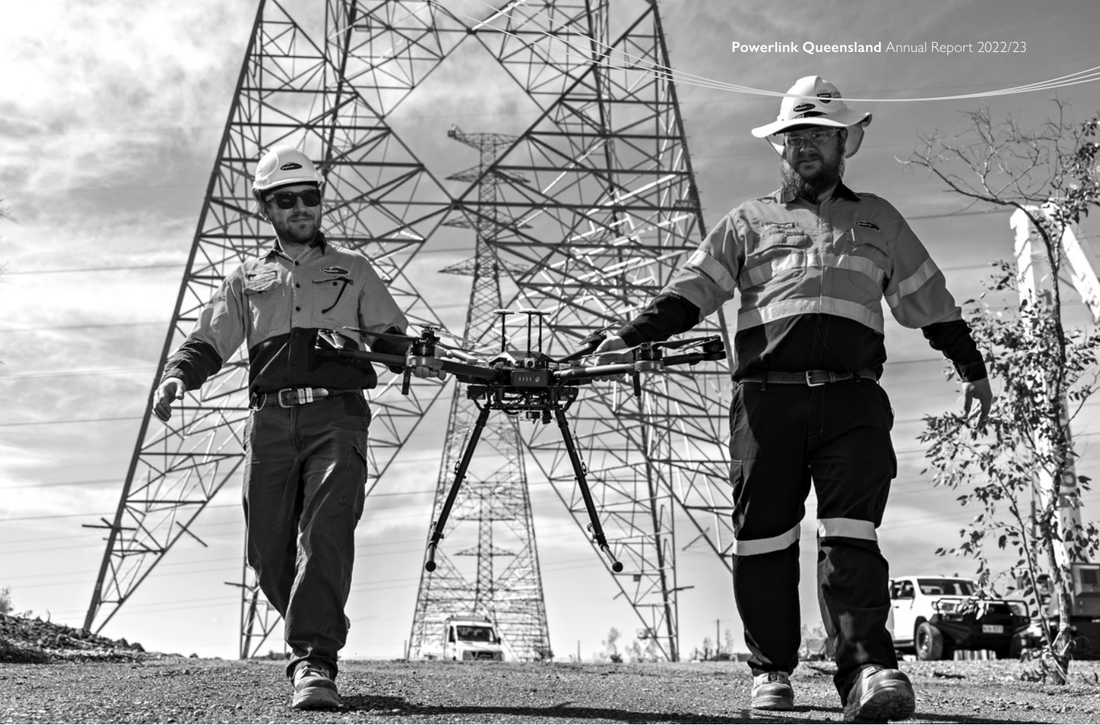
Launching a drone used for line stringing of the tallest towers on our transmission network in Far North Queensland.
