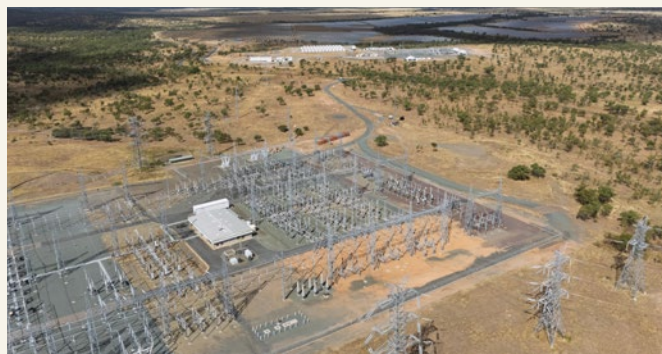
Powerlink's connection to Iberdrola's Broadsound Solar Farm is now complete.
