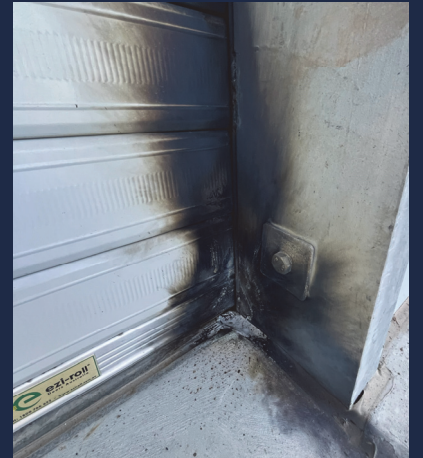
i Nearby warehouse damage
