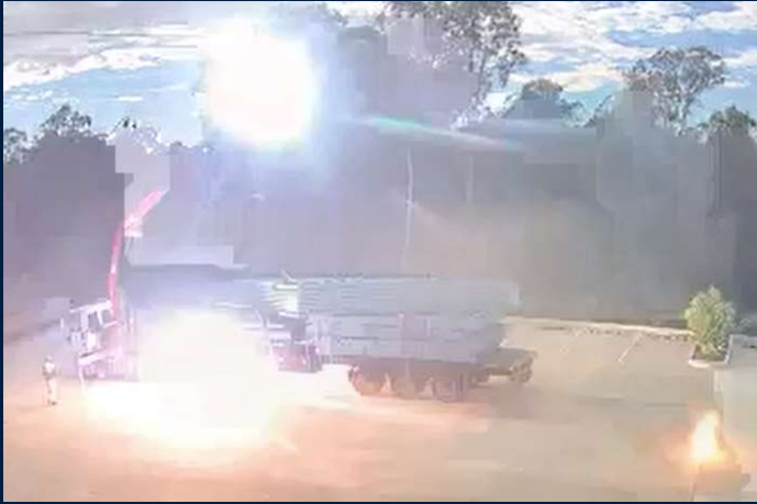
i Vehicle-mounted crane operated within the exclusion zone of 110kV powerline
