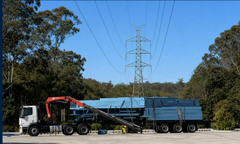
i Work location directly under powerlines
