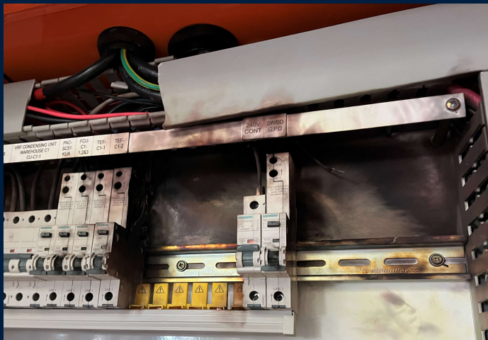
i Nearby warehouse switchboard damage
