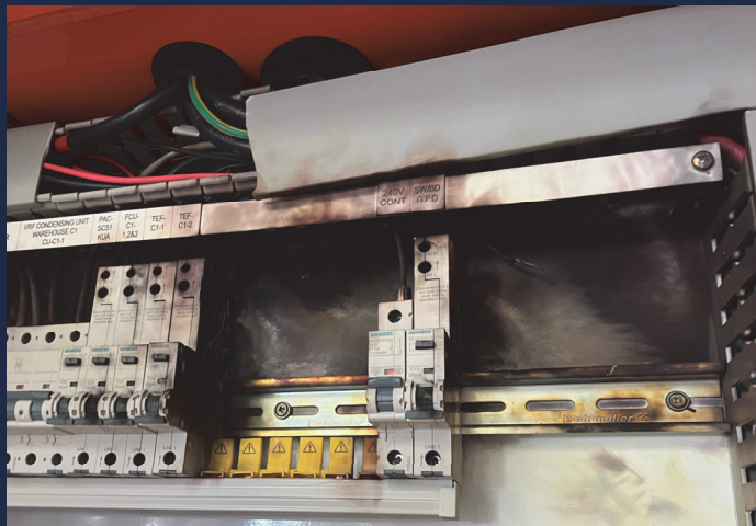
i Nearby warehouse switchboard damage
